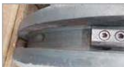
Steam Joint Damage
