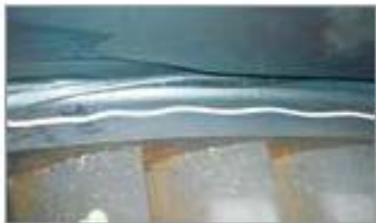
Diaphragm Body Damage
