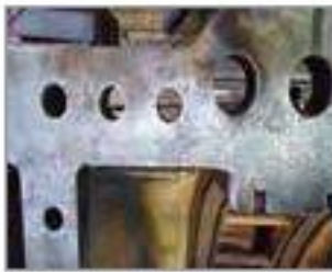
Casing H/J Damage
