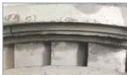
Spill Strip Damage
