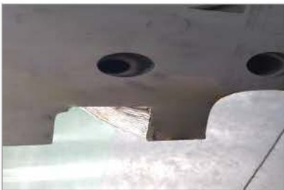
Horizontal Joint 손상
