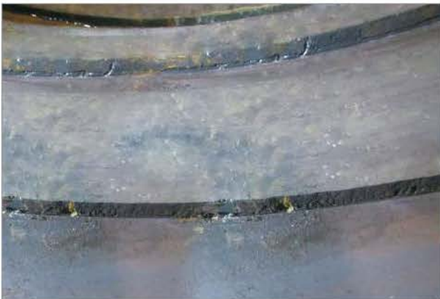
BFPT Casing Seal Face 손상
